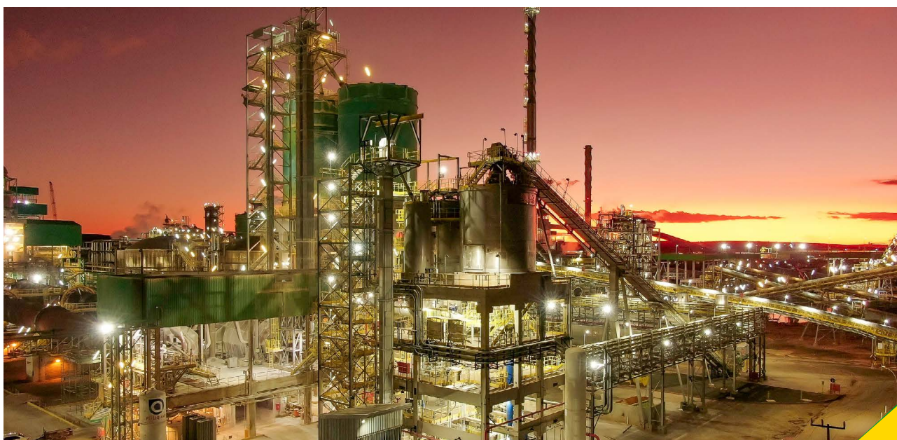
Biomass gasification plant at the Ortigueira Unit (Paraná)
